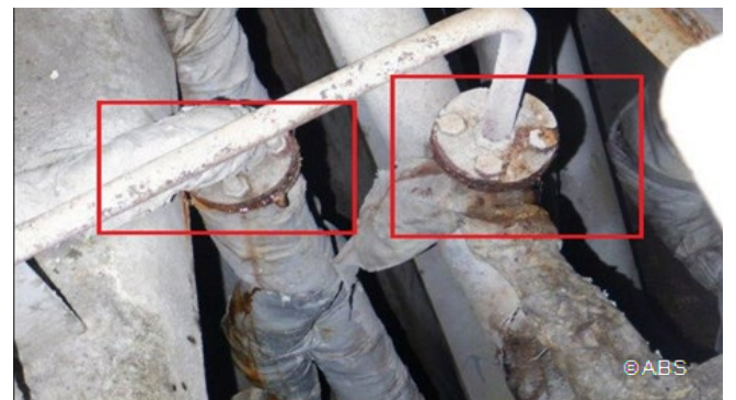
Steam pipe leaking
