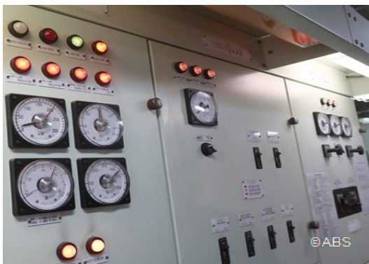
Numerous Indication lights on emergency generator panel out of order
