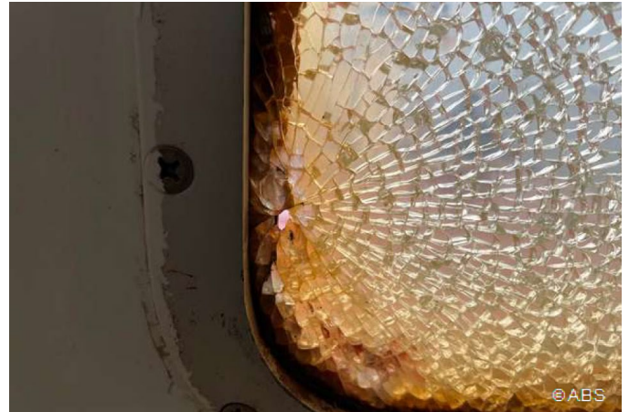
Accommodation window shattered with hole
