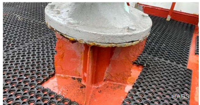
Bridge Wing Compass Pedestal wasted
