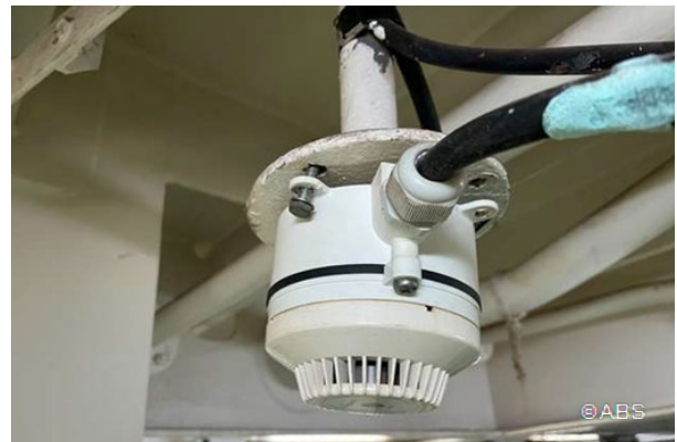
Fire detector not secured in the base
