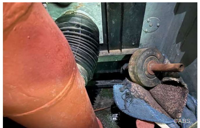
Sewage System Flexible pipe leaking
