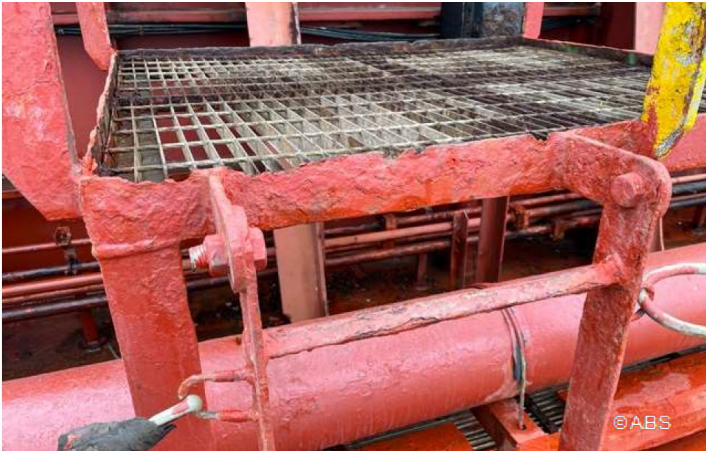
Standing platform excessively wasted
