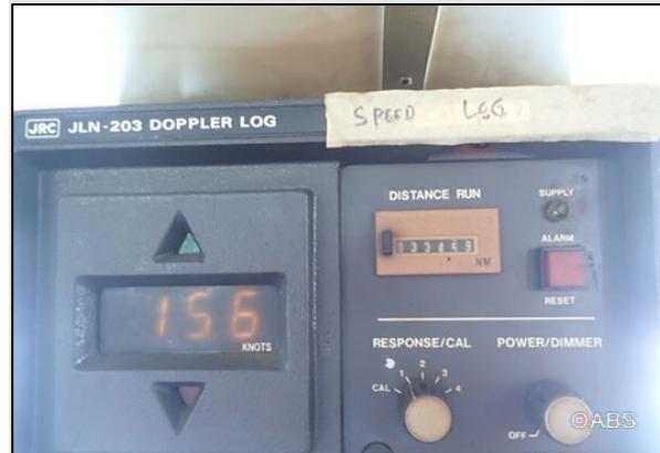
Defective speed log, showing speed on vessel at anchorage
