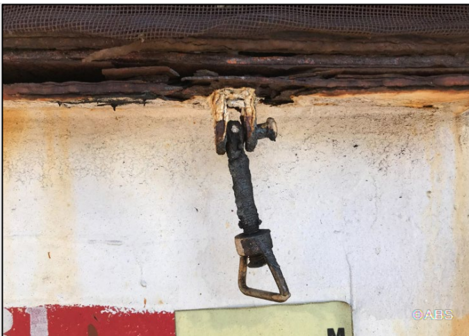
ER ventilation damper with damaged dog and corroded coaming
