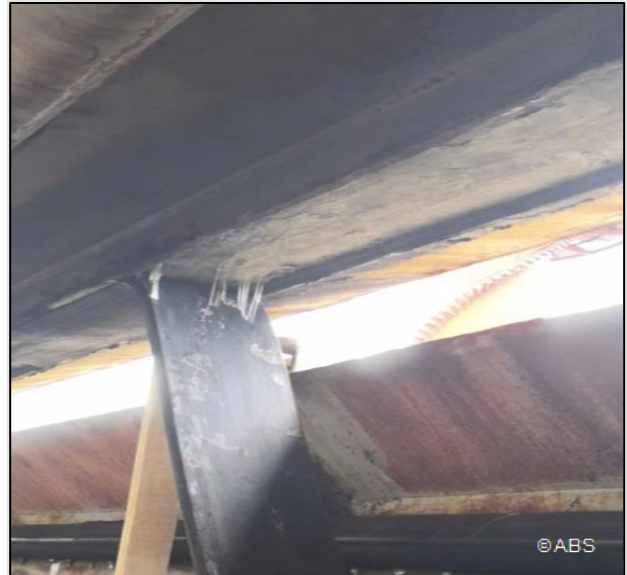
Rubber packing of cargo hatch cover missing and or damaged
