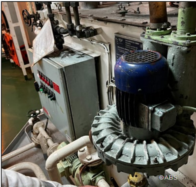
Sewage treatment plant not operable
