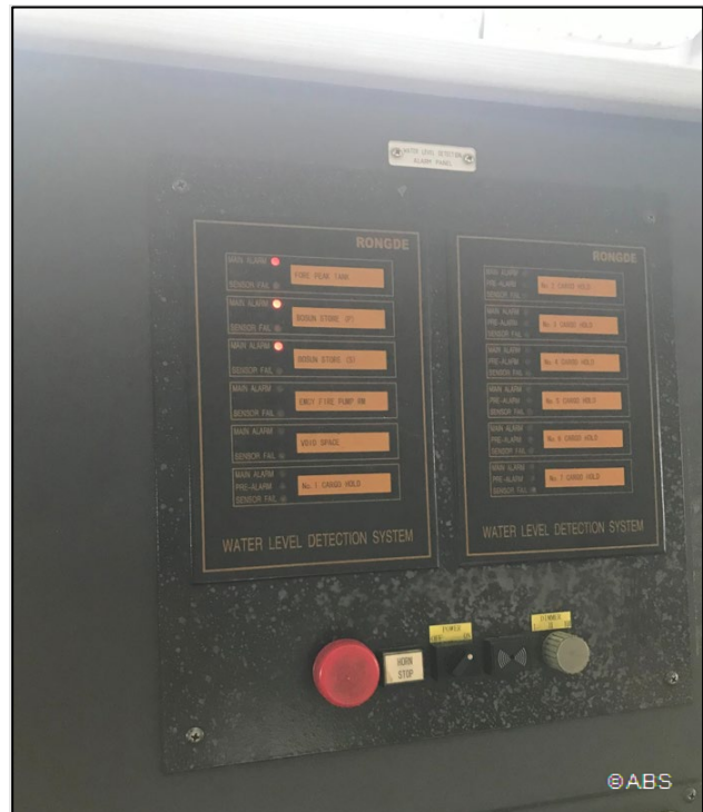
Water ingress alarm system defective
