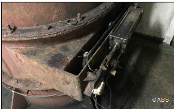
ER fire damper unable to operate (close)
