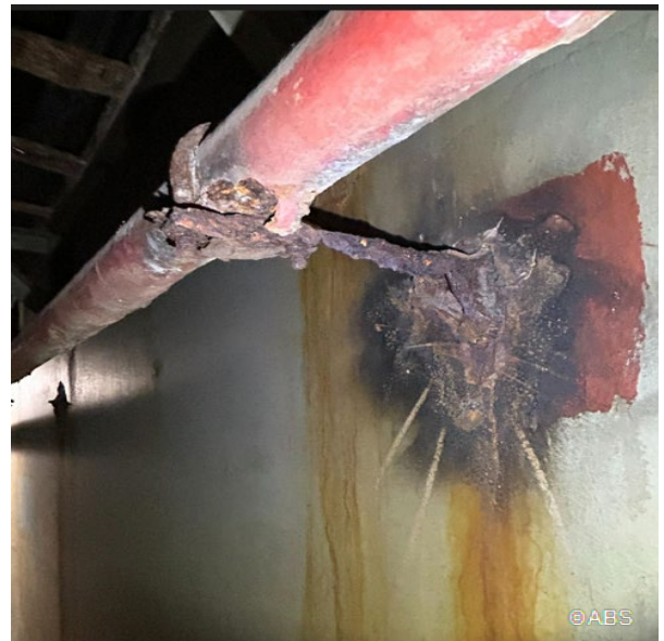
Fire main support wasted
