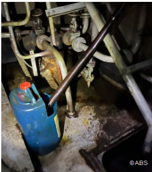
Unapproved modification in engine room bilge line above tank top
