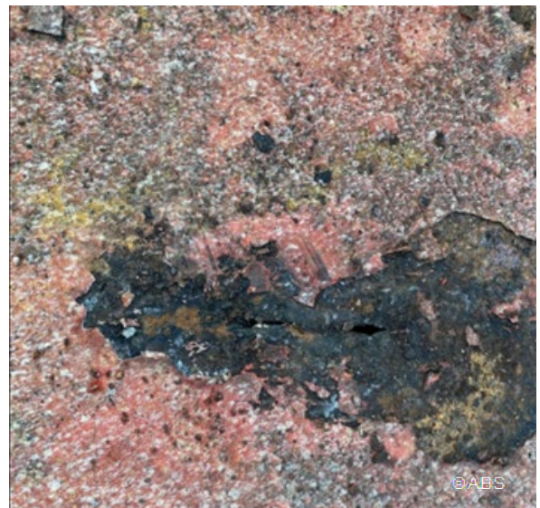
Main deck wasted with hole, next to hatch coaming in a bulk ship
