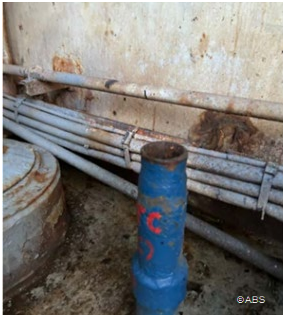
Sounding pipe securing thread wasted
