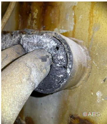
Cable transit compound damaged and found with hole at cargo hold tunnel
