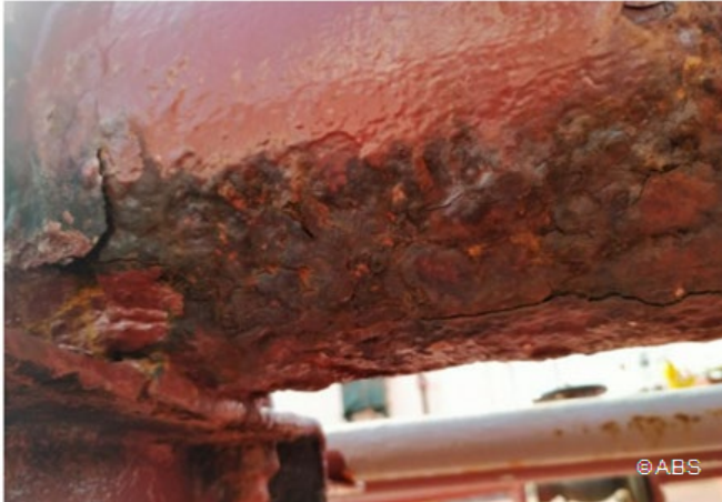
Excessively wasted pipe and support located at main deck
