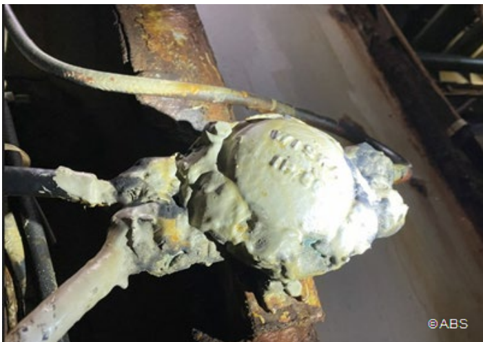
Electrical junction box not maintained
