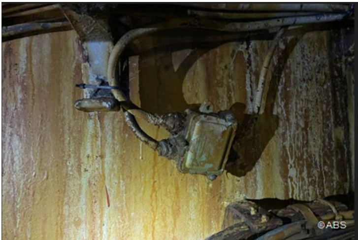
Electrical cable not maintained in tunnel
