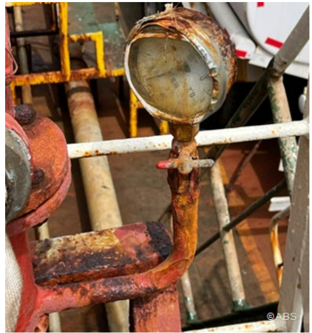
Faulty and damaged fire line pressure gauge
