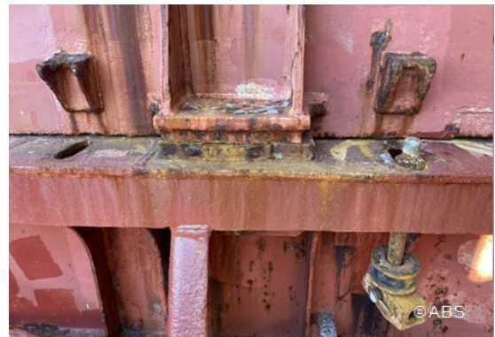
Cargo hold securing devices worn, missing securing wingnut, not able to secure hatches
