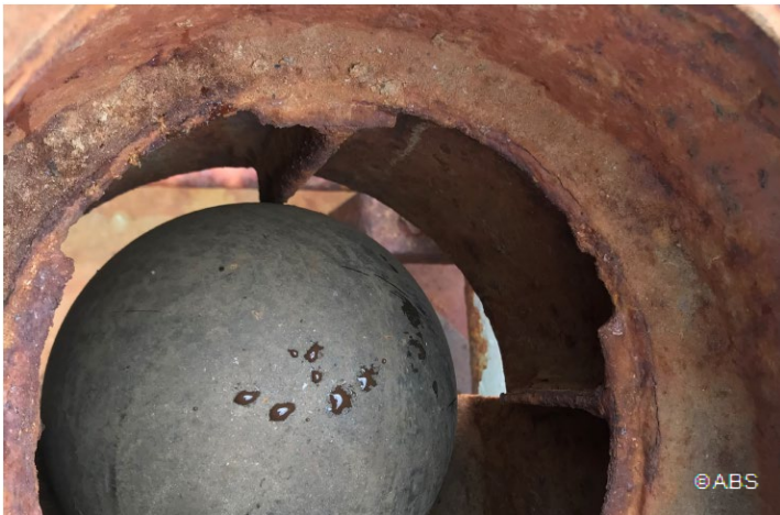
Tank vent head ball is stuck and not making positive seal, due to damaged structure
