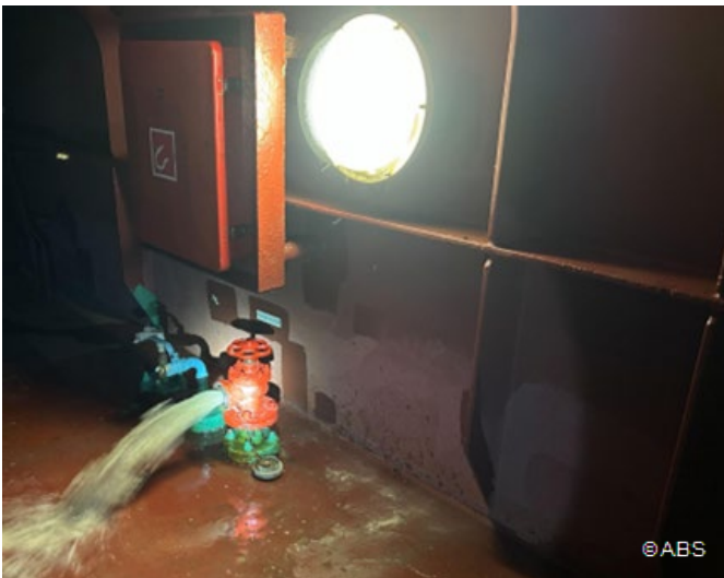
Leaking fire hydrant due to isolation valve leakage
