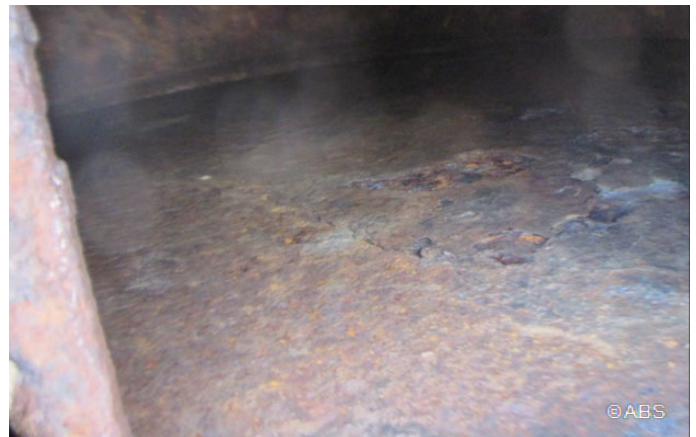
Fire damper for ER ventilator wasted and seized in position
