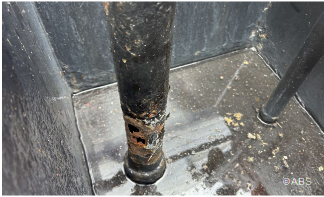
Emergency generator fuel oil tank, air vent pipe wasted with holes and covered with tape
