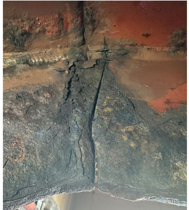
Cargo hold coaming stiffener fracture
