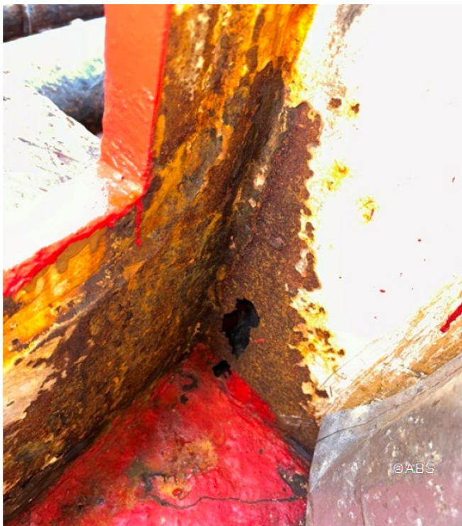
Emergency escape to main deck from engine room, structure wasted with holes
