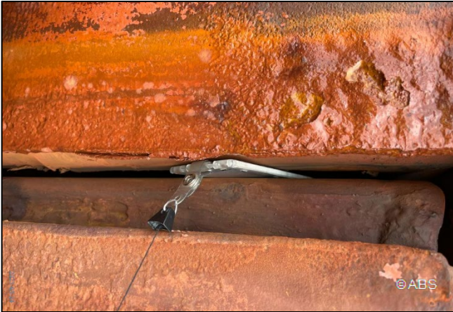
Cargo Hold hatch cover is not weather tight in closed position
