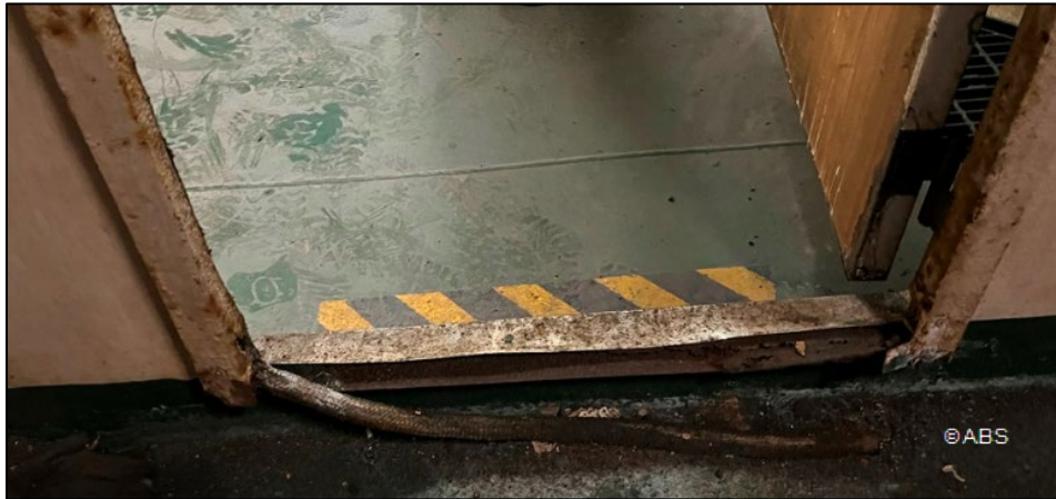
Fire door seal damage
