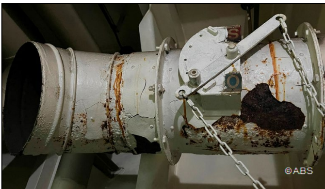
Wasted blower duct, inoperable flap
