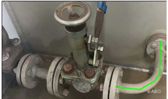
Emergency diesel generator quick closing valve-fitted with 250mm apart from tank, does not meet requirement
