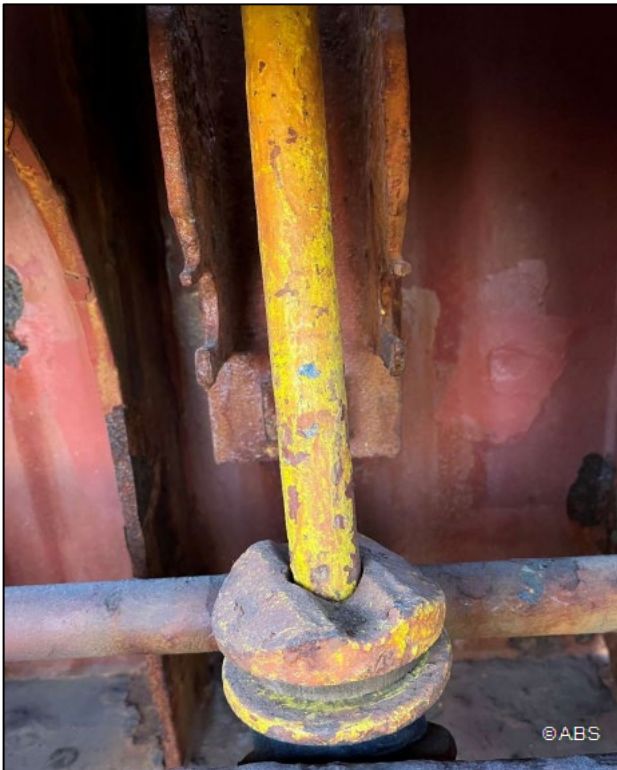
Cargo Hold Cleat securing arrangement wasted and detached
