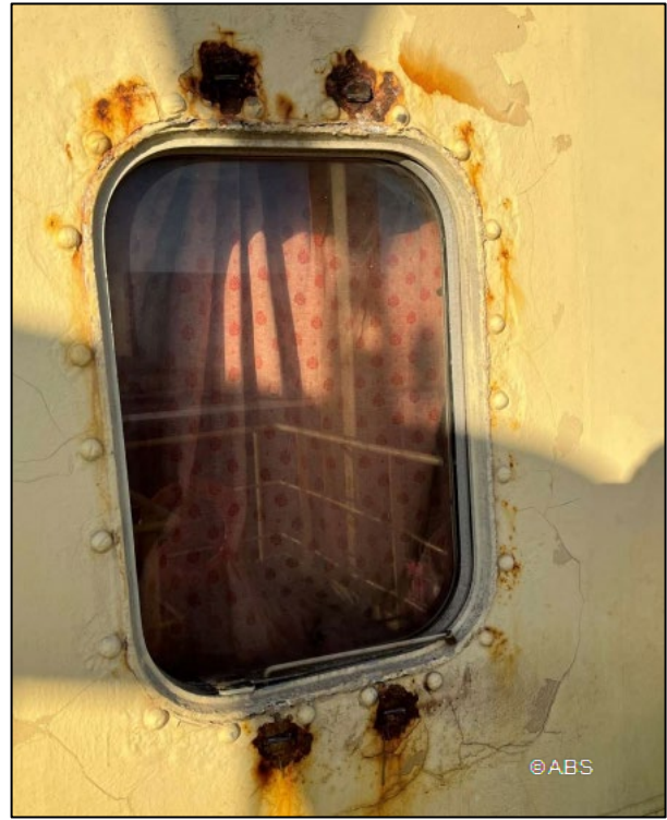
Safety bar missing from accommodation window
