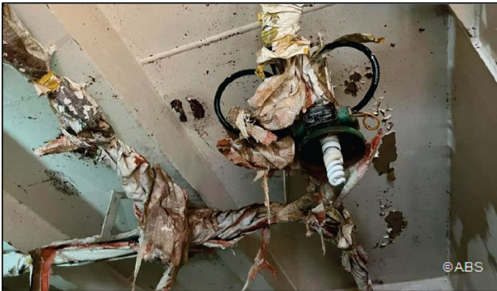
Insulation damage, electrical fixtures not maintained
